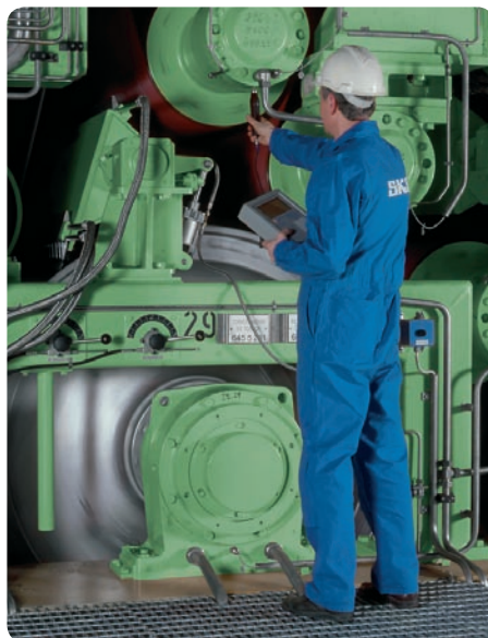
Checking vibration levels
